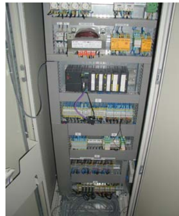
Besturing (PLC Siemens S7)
